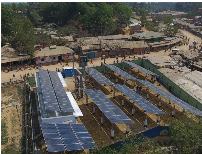
The biggest solar-powered water supply system of the Rohingya crisis, installed in Camp 12, Cox's Bazar, Bangladesh. © IOM 2018
